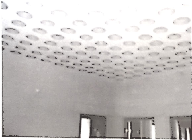
A house built with SMB walls and filler slab roof using earthen pots
